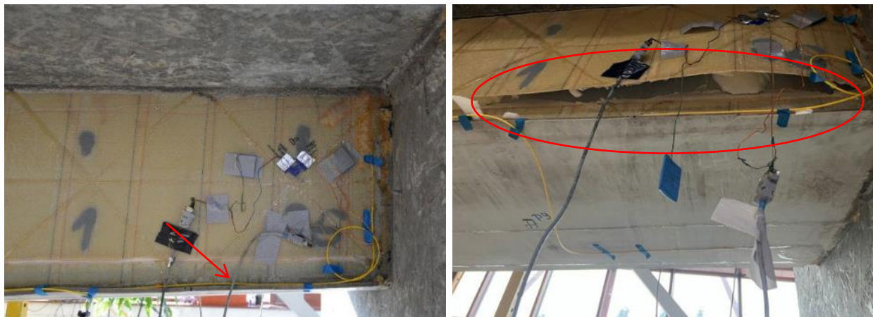
Figure 7. The support zone in the lower depth end of the girder (left) and the failure mode (local fracture) of the shear web in this support zone (right)
